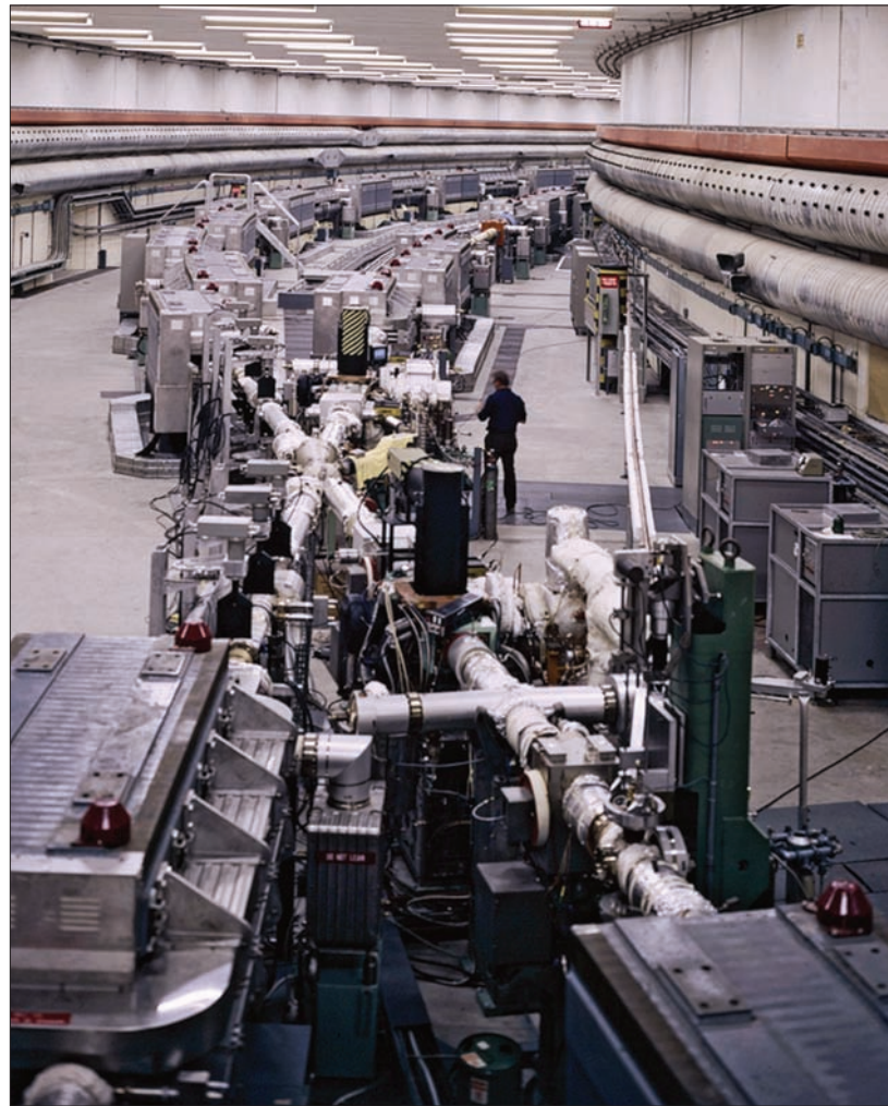
This view of Intersection 5 (I5) in 1974 clearly shows the layout of the magnets and the crossing of the two beam pipes.
